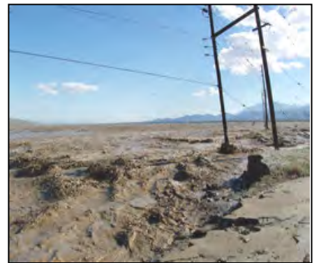
Flooding along Indian Canyon Drive, January 11, 2005.
