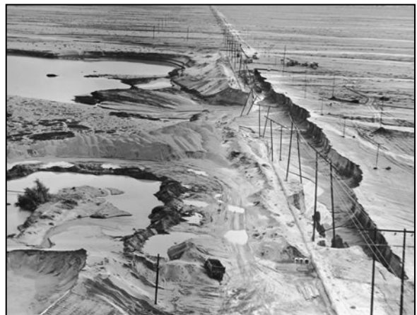
Flood damage to Indian Avenue by the 1965 Whitewater River floodwaters caused the road to be closed for 30 days, adding to the isolation of Palm Springs. (Source: RCFCWCD)
