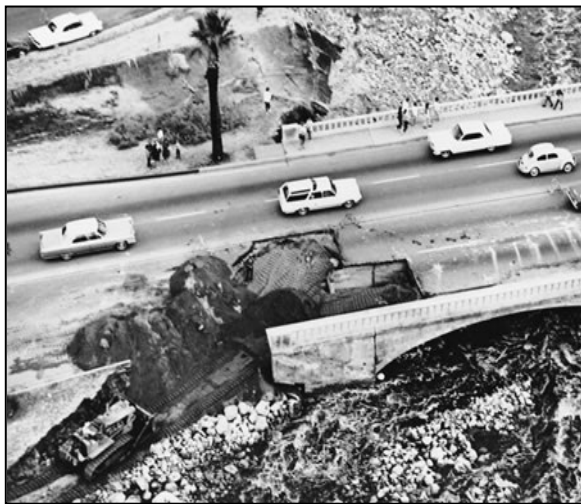
Flood damage to Highway 111 from 1965 storms.
